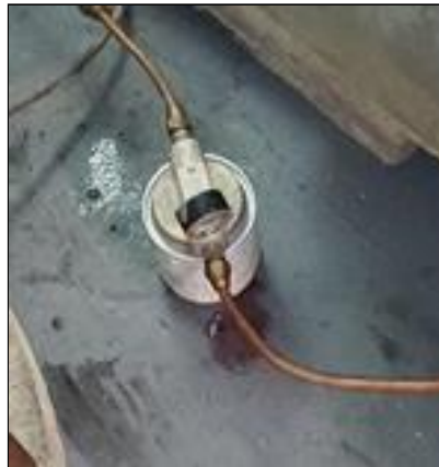
7.0 Item 2(Picture) oil furnace in the basement component appears to be leaking, and is not secured
