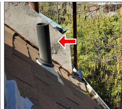
5.3 Item 5(Picture) Example/ Sample- Rear of home-
