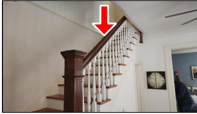
3.4 Item 1(Picture) Example/ Sample- handrail height to low
