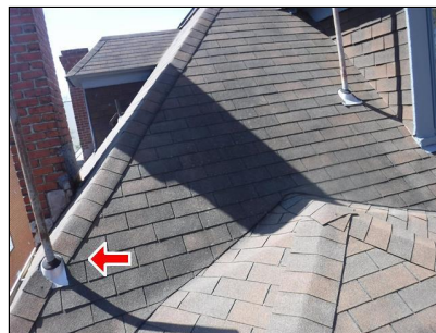
1.0 Item 6(Picture) Example/ Sample- pipe penetrations in valleys and/or ridges considered unconventional however a typical finding on a structure of this age potential for roof leaks are higher
