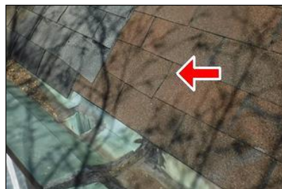
1.0 Item 3(Picture) Example/ Sample- front of home shingle loose and or installed improperly
