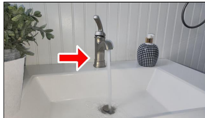
5.4 Item 4(Picture) Example/Sample- First level Hall Bathroom Sink- faucet loose at countertop
