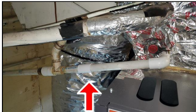
7.0 Item 5(Picture) Example/ Sample- condensation line for AC in the basement missing recommended TRAP – condensate may not drain properly
