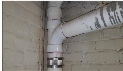
5.3 Item 3(Picture) Plumbing leak appears to be coming from pipes above this area
