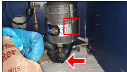
5.4 Item 3(Picture) Example/Sample- Kitchen Sink- P-trap cleanout not accessible, Plumbing leak(s) observed.
