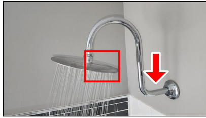
5.4 Item 9(Picture) Example/ Sample- Primary Bathroom Shower- shower supply pipe is loose, shower heads leaks while in use
