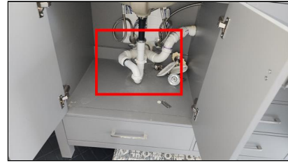
5.4 Item 11(Picture) Primary Bathroom Left Sink has unconventional plumbing
