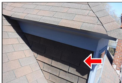
1.0 Item 1(Picture) Example/ Sample- shingles on one or more dormers considered lifted risen this is a common finding due to during insulation installers not apply sealant on the tabs – prone to be blown off for example during periods of high wind
