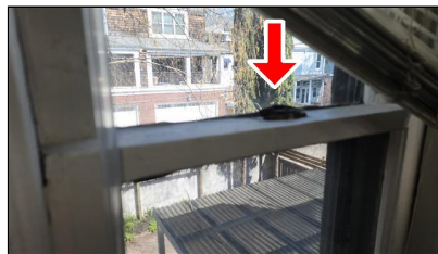
3.6 Item 3(Picture) Example/ Sample- Second level Hall Bathroom- Did not latch/lock
