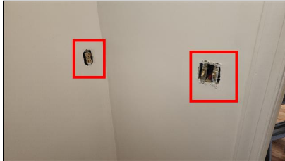
6.5 Item 1(Picture) Example/ Sample- Third level unfinished Wash Room- cover plate missing
