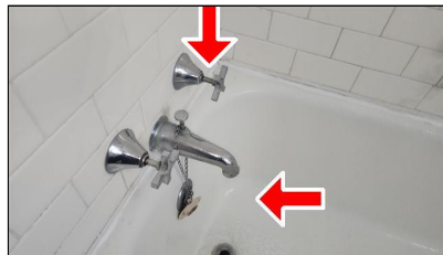
5.4 Item 7(Picture) Example/Sample- Second level Hall Bathroom Shower- tub spout leaks when in shower mode, water control handle leaks while in use
