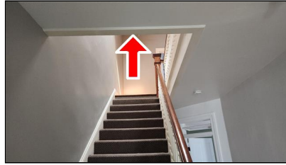
3.4 Item 2(Picture) Example/ Sample- height clearance inadequate
