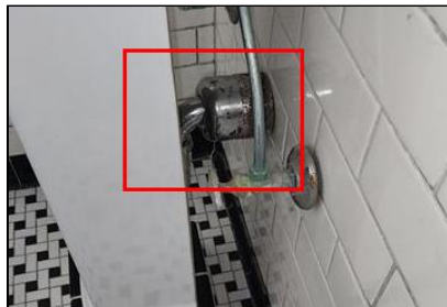
5.4 Item 6(Picture) Example/Sample- Second level Hall Bathroom Sink- chrome waste piping is susceptible to leaking
