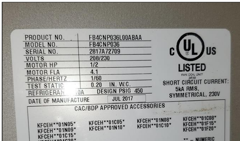
air handler label located 3rd level side attic access –CARRIER – manufacture year 2017
