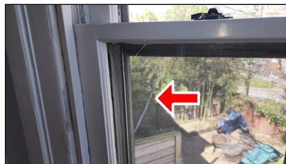
3.6 Item 6(Picture) Example/ Sample- Second level Rear Bedroom- Damaged glazing/glass
