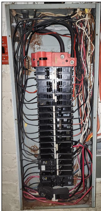
6.3 Item 1(Picture) Electrical panel(s) uncovered by inspector during inspection
