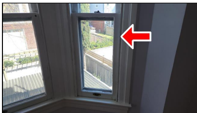
3.6 Item 5(Picture) Example/ Sample- Second level Rear Bedroom- Stuck shu
