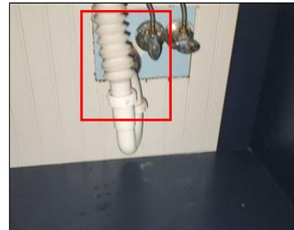
5.4 Item 5(Picture) Example/Sample- First level Hall Bathroom Sink- corrugated drain line, leak observed
