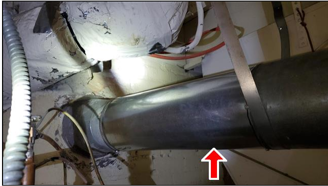
7.0 Item 3(Picture) Example/Sample- vent pipe for oil type not confirmable due to label missing and or not observed by inspector
