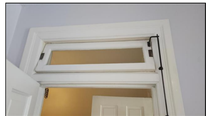
3.6 Item 4(Picture) Example/ Sample- Second level Rear Bedroom- Pass thru windows that are above bedrooms are not tested during inspection
