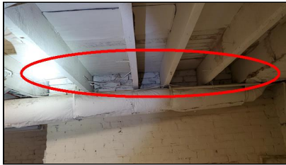
4.0 Item 1(Picture) Example/ Sample- floor joist do not have the recommended airspace upon entering/resting into the Masonry wall which is typical for the age of structure. However this hampers inspection of the wood members
