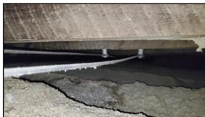
6.4 Item 7(Picture) Example/ Sample- attic – tested not active however recommend remove
