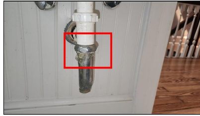
5.4 Item 10(Picture) Example/ Sample- Third level Hall Bathroom Sink- leak observed
