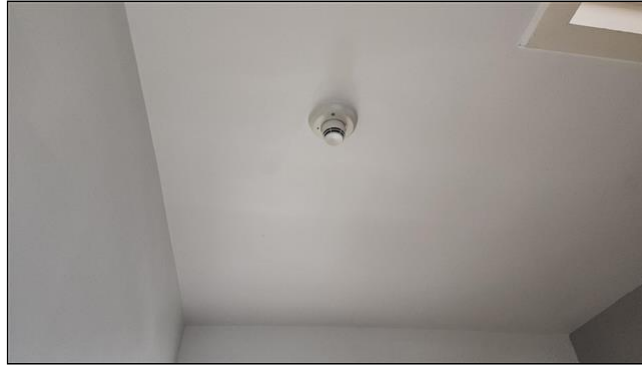
6.11 Item 2(Picture) Example/Sample- Second level Hallway- aged
