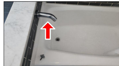
5.4 Item 8(Picture) Example/Sample- Primary Bathroom Shower- tub spout plumb supply pipe is loose
