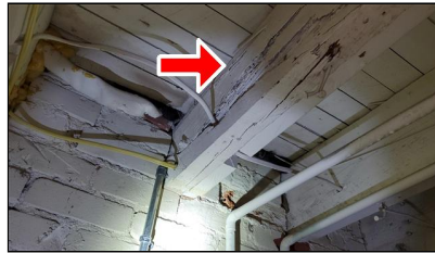
4.0 Item 2(Picture) Example/ Sample- floor joist – deteriorated/ damaged wood member(s)
